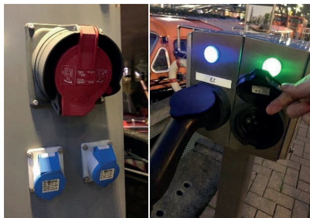
Figure 9: Simple industrial socket chargepoint and Type 2 chargepoints for both e-boats
