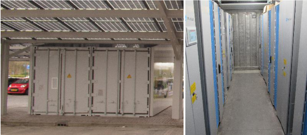
(a) Battery housing located under the carport roofs (b) Battery cabinets within the housing
