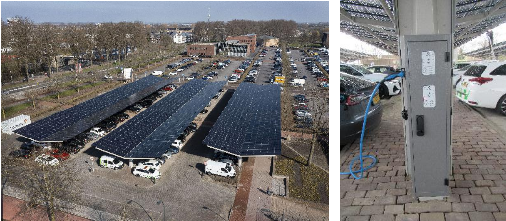
(a) PV array at the solar parking lot located at the municipality building of Dronten, the Netherlands (b) Charging station with 4 charge points
